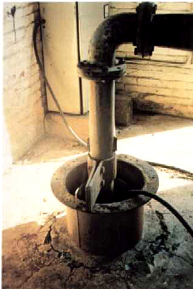
Plate 17.1: Groundwater bores should be protected to prevent contamination. Here the concrete around the bore is cracked and the top is open, increasing the risk of pollution.
